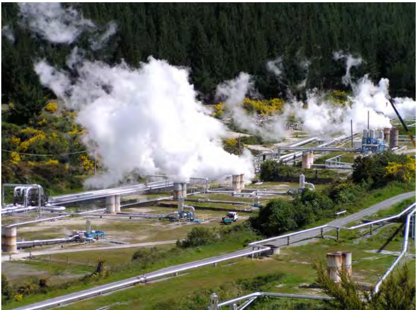
Geothermal plant in Wairakai (New Zealand) Photo: Geothermal Resources Council
